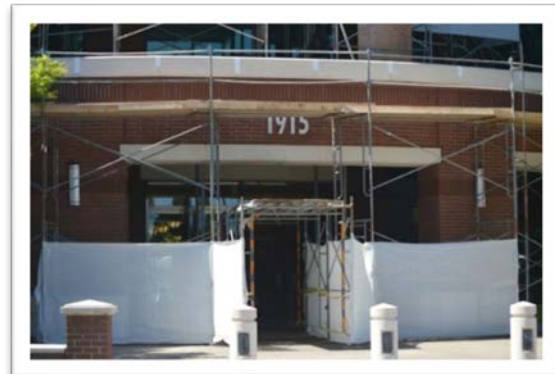
Figure 4: Proper attempt at securing cross bracing with wire.
