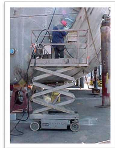
A scissor (or aerial lift) may be regarded as a suspended scaffold.
