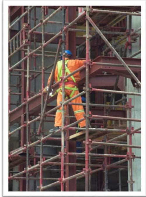
The worker in this picture is using fall protection to prevent accidents.
