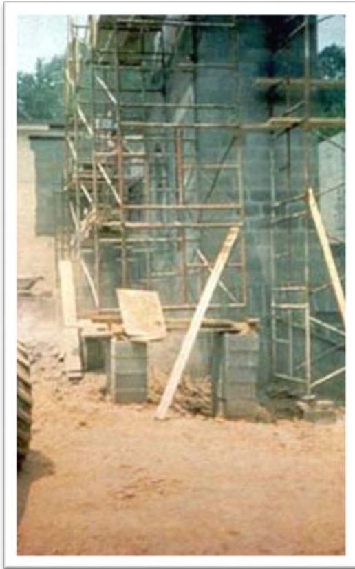
Figure 1: Poor foundation-Shows scaffold end frames, which have no base plates, erected on the top of scrap wood and unstable cement blocks.
