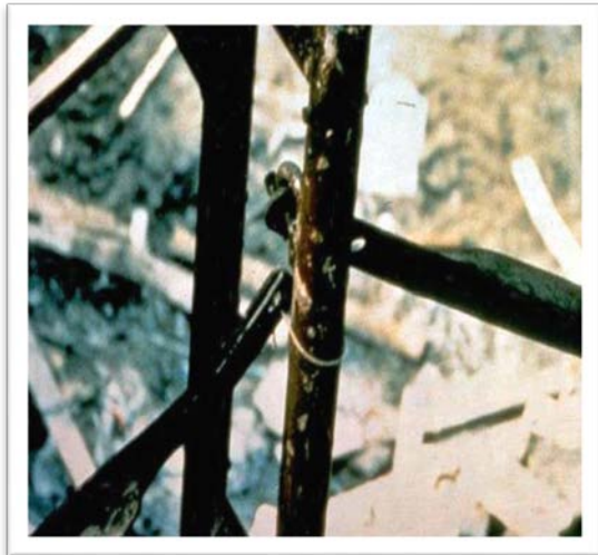
Figure 3: Poor attempt at securing cross bracing with wire.
