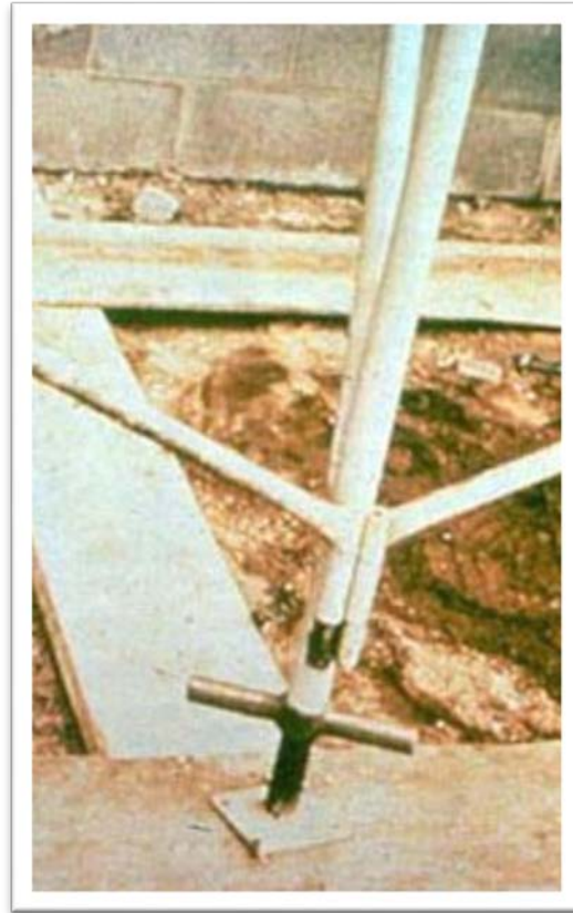
Figure 2: Proper foundation- Shows scaffold end frames equipped with adjustable screw legs and with base plates set on mud (wood) sills.
