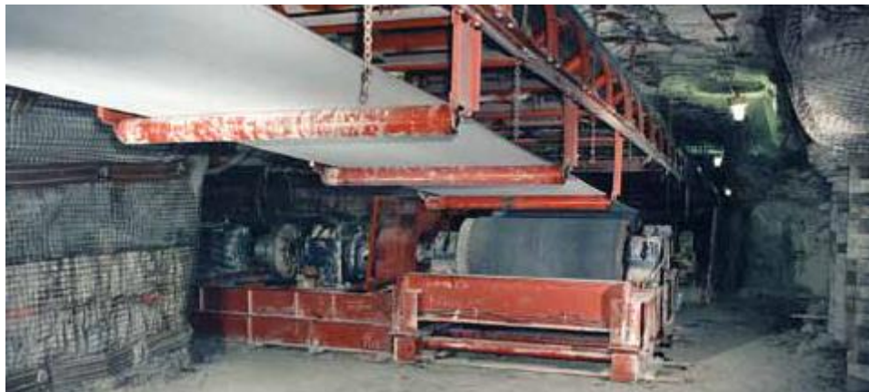
Figure 48. Typical rigid-frame belt conveyor set-ups for a CM section and main line (Grayson, 2014)
