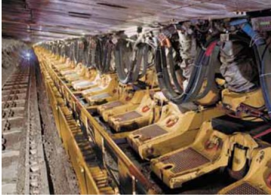
Figure 66. Installed CAT longwall system. (Grayson, 2014)
