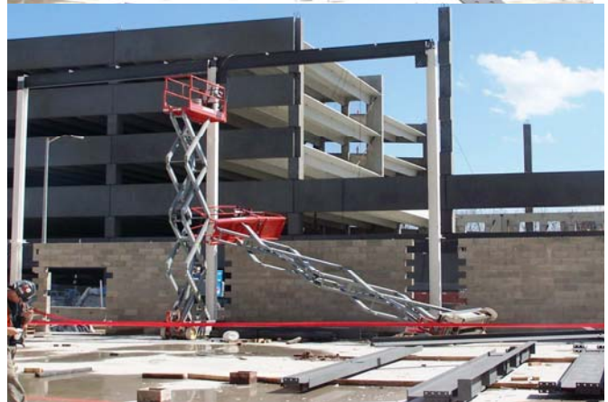
Picture of the complete work area with lift blown over.
