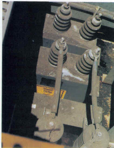
PCB marked capacitors in a coal mine power center.
