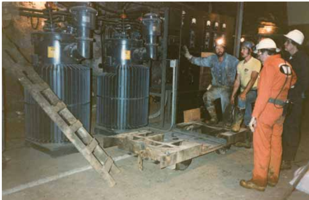
Fig. 2 76-gallon PCB (Pyranol) transformers in the Eagle Mine at Gilman, Colorado
