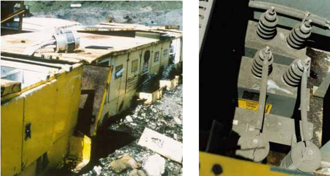
Fig. 6 Coal mine power center containing PCB capacitors
