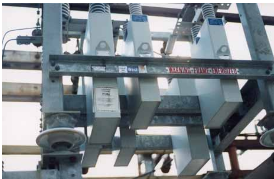
Fig. 3 Marked PCB capacitor on the left
