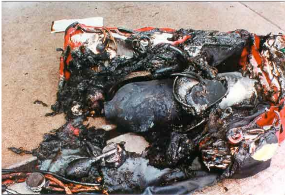
Photo 2: This photo depicts the damaged oxygen system
