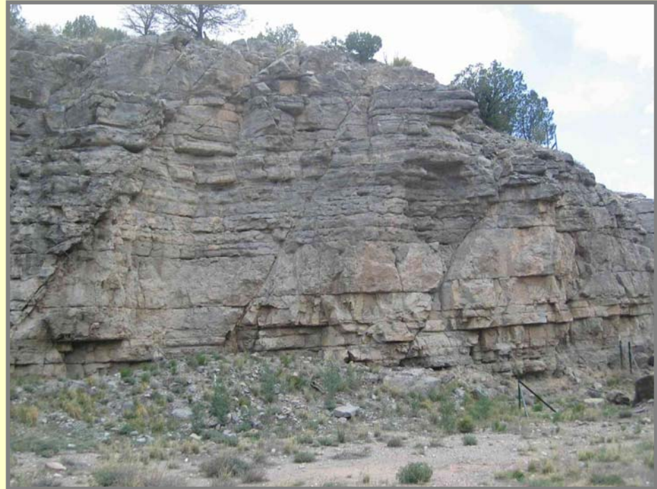
Highwall cut showing horizontal bedding planes cut by inclined joints that offset beds in the limestone.
